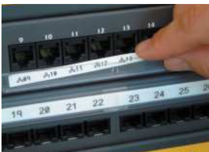
Punch block & patch panel labels
